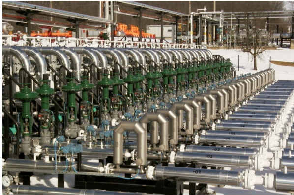
Figure 10. Natural Gas Storage Management Using Coriolis Meters
